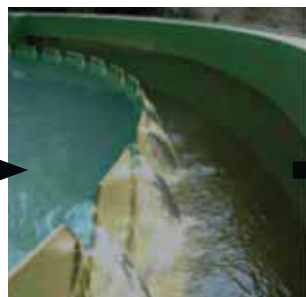
Water separating from sludge
